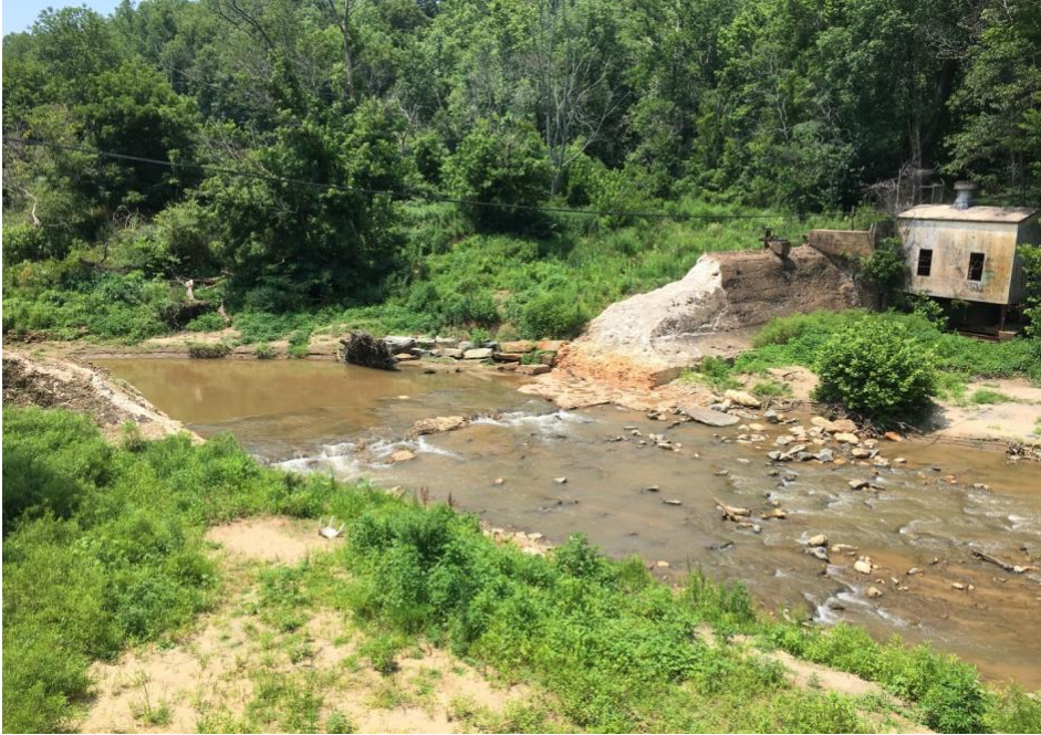
Figure 2.3.2 – July condition of dam on Power Dam Road after removal. Legacy sediment appear to be a continual problem. Note the discoloration of the water even during low flow conditions.
